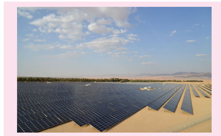
צילום: APC- Arava power company
